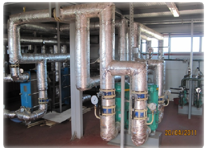
Figure 1. Modernized boiler house in Luschik village of Bezhanitskiy Rayon (inside view)
